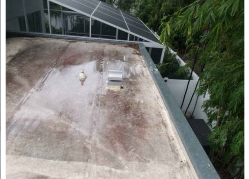
Plumbing vent and exhaust fan vent from master bathroom
