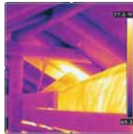
Above - Leaking ductwork is heating up the framing around the area.
