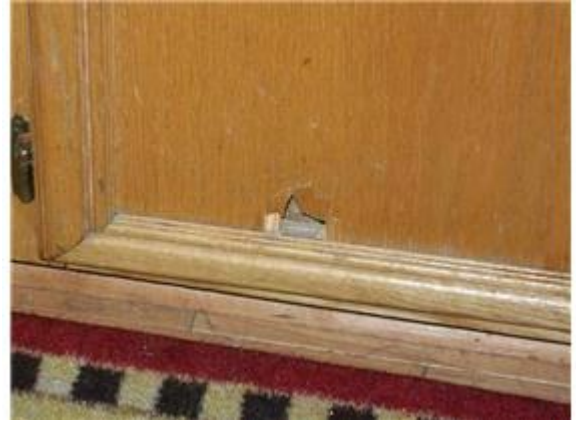
Damaged kitchen cabinet door
