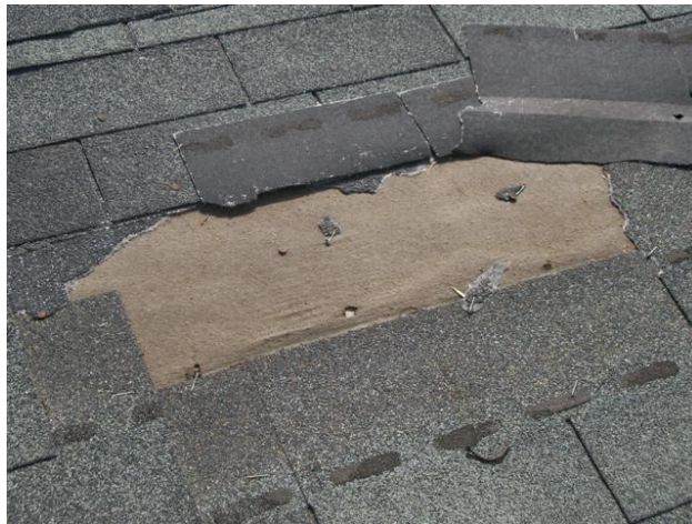
Additional damaged area
