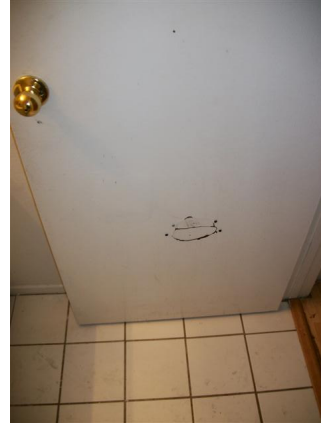
Damaged bathroom door
