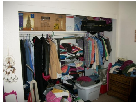
Missing closet doors
