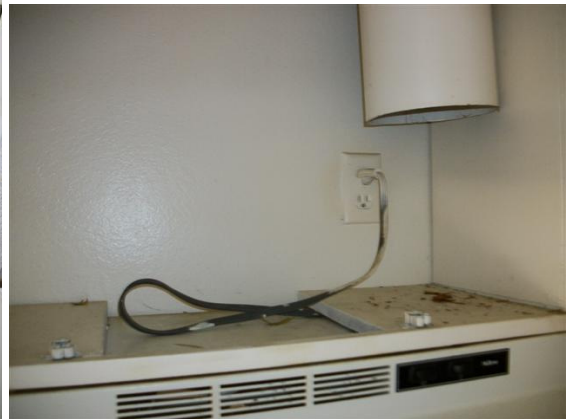
Improper exhaust venting
