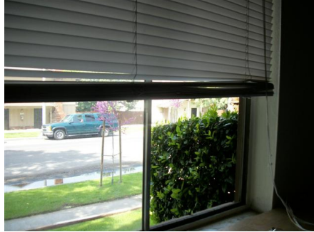
Missing window screen
