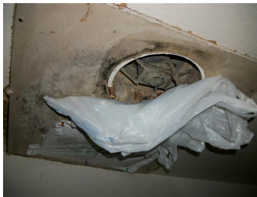
Bathroom ceiling damage
