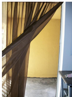
Missing window screen
