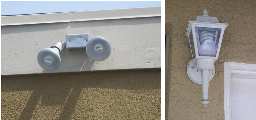
Exterior light fixtures
