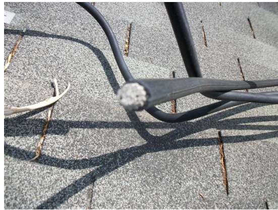
Exposed service drop
