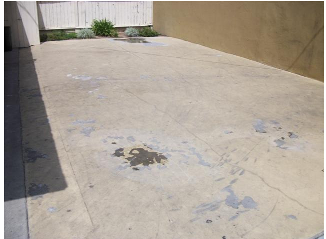
Pooling on slab
