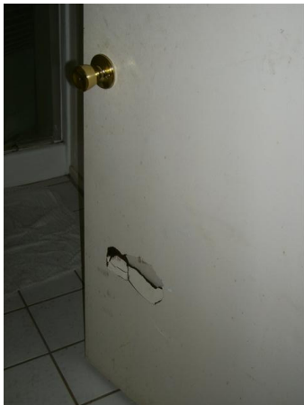
Damaged interior door
