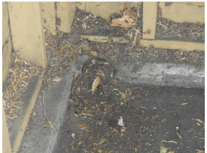
Obstructed drain line in carport
