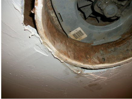
Plumbing leaks above ceiling
