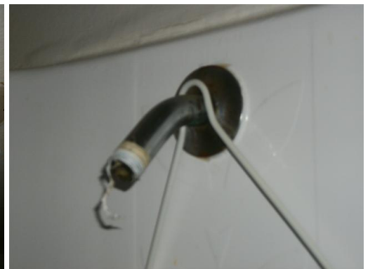
Missing shower head
