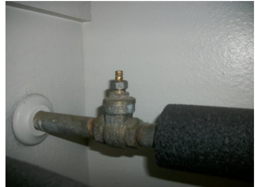
Missing valve at water heater
