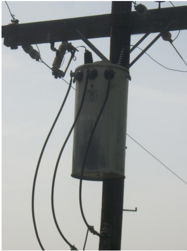
One of two pole mounted transformers
