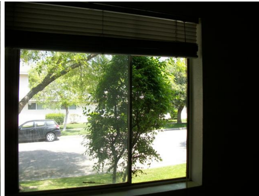
Missing window screen
