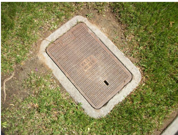
View of water meter
