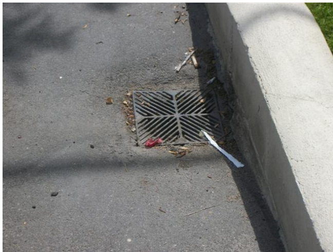
Slow drain in parking lot
