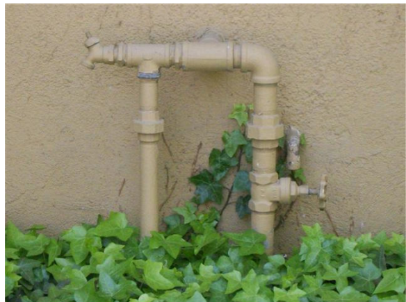
View of one of the water valves
