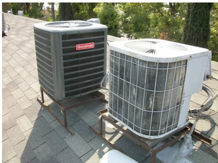
View of condensers
