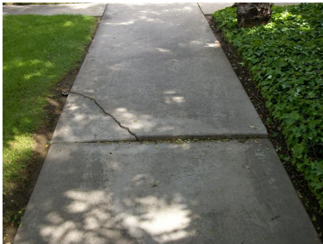
Damaged sidewalk – trip hazard
