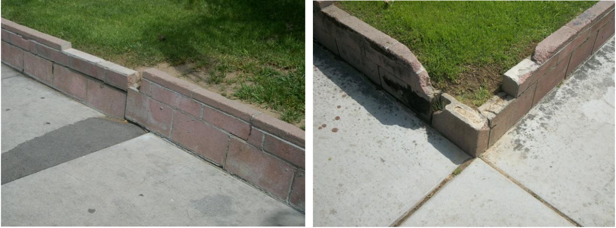
Damaged areas of the retaining wall
