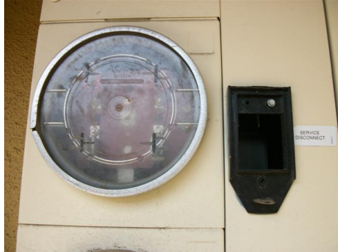
Missing electrical meter
