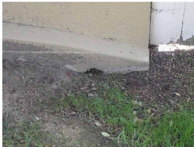
Dirt needs to be graded back from drain opening
