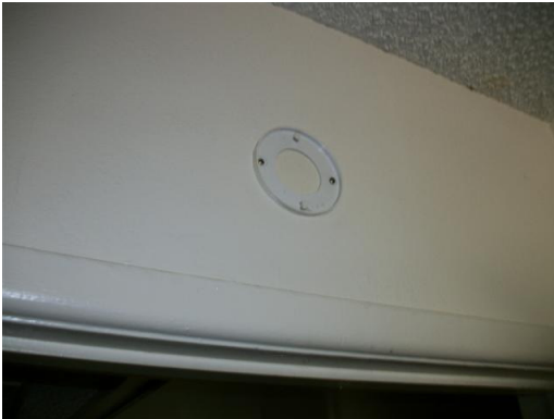
Missing smoke detectors
