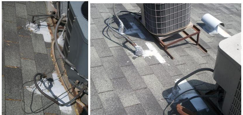
Missing insulation from lines
