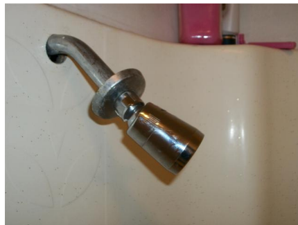
Shower head weak water pressure
