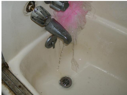
Tub faucet dripping
