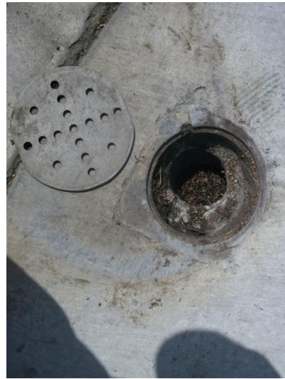
Clogged drain line on walkway
