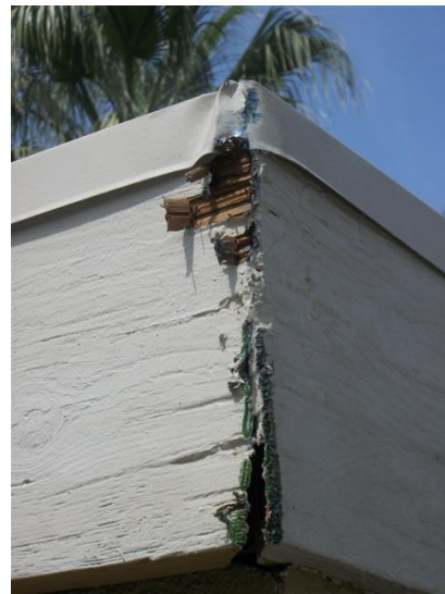
Dry rot wood damage
