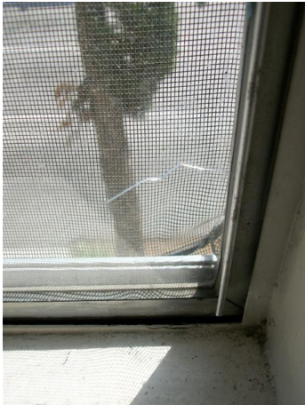
Cracked window pane
