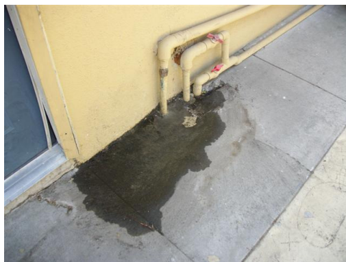
Additional leaks at pool supply line
