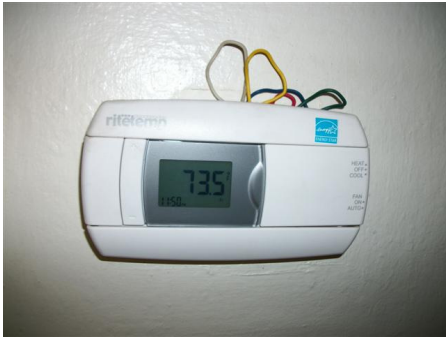
HVAC system not operable
