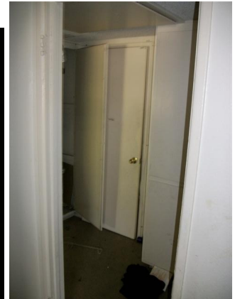
Missing interior door
