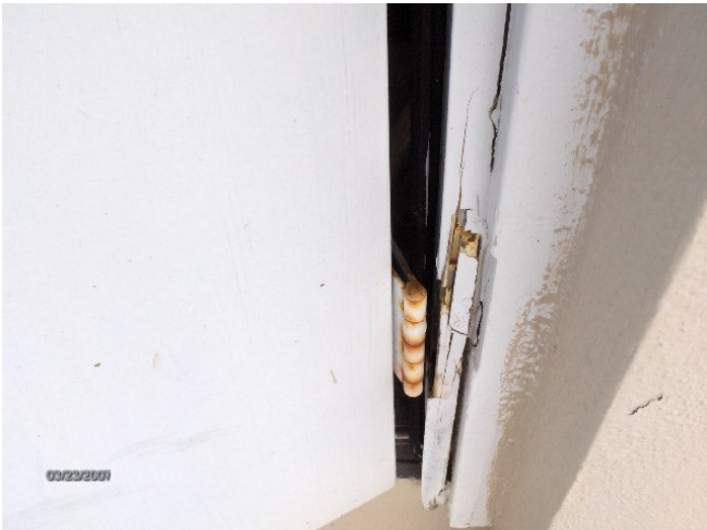
Damage to door and door jambs at garage utility door.
