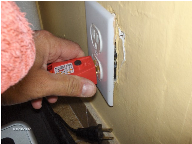
Outlet in master bedroom bathroom is very loose from wall.
