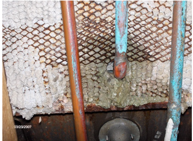
Severe water leak at main bathroom shower access panel.
