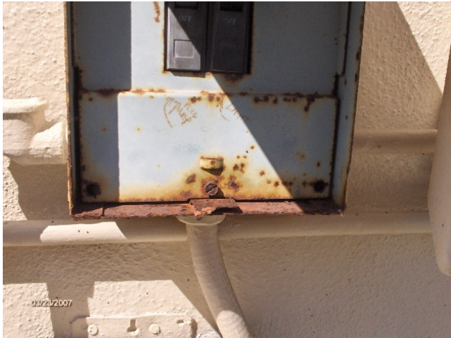
Pool electrical panels rusted and damaged.
