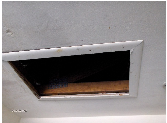
Recommend replacing attic access cover in garage.
