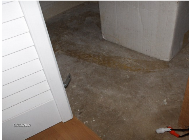
Floor not complete inside closet of west side bedroom.
