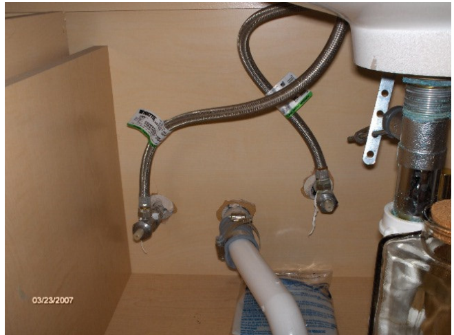
Bathroom sink faucet shut-offs missing their handles.
