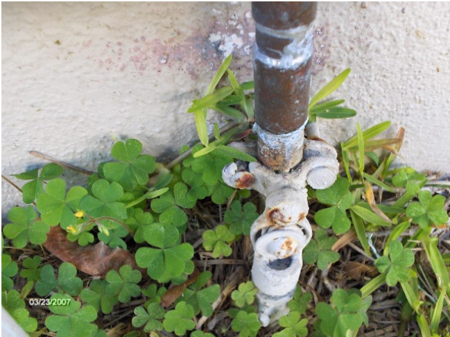
Bond clamp loose at water main.
