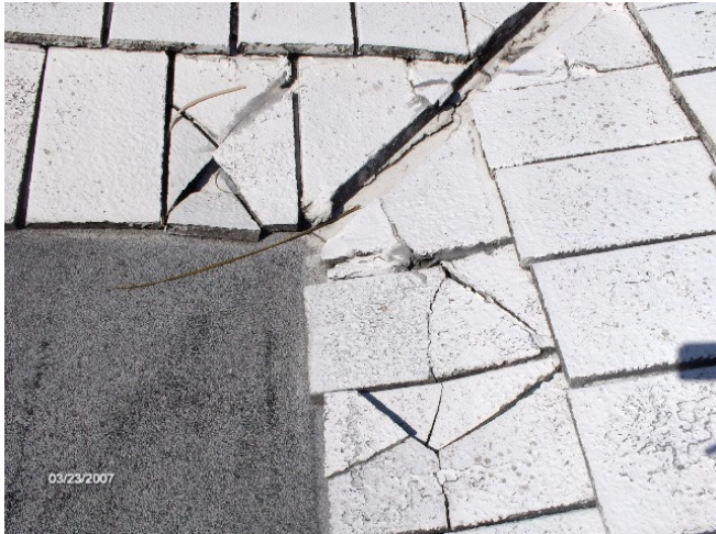
Several broken/cracked/detached roof tiles at most areas of the main roof.
