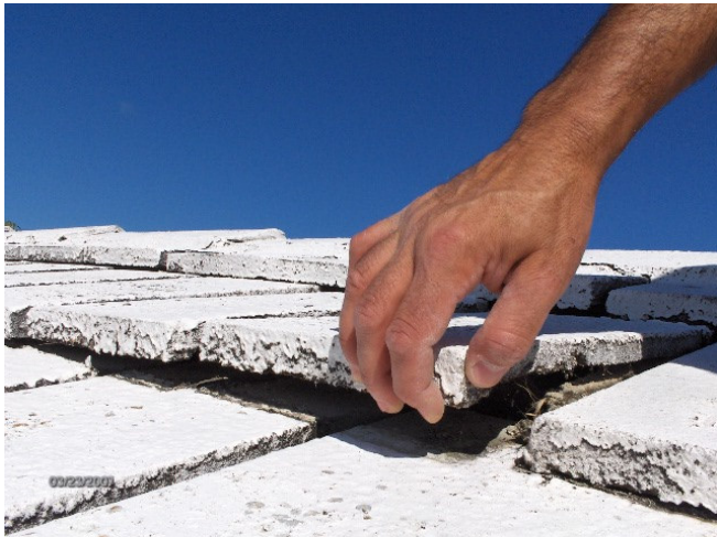
Loose roof tiles present.
