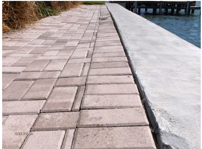
Sunken area of paver walkway above seawall/below pool.
