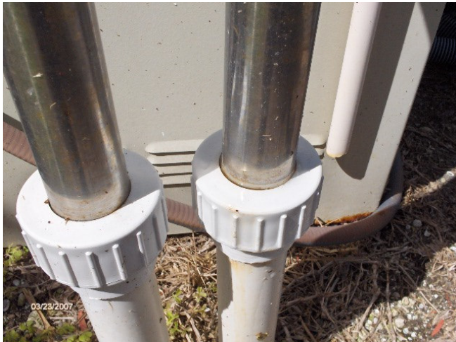
Leak at output line of pool heater.
