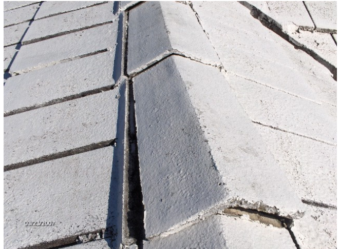
Detached and broken roof tiles at peaks.
