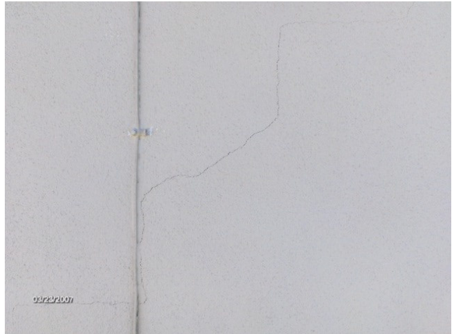
Hairline "step" cracks at s/w corner of stucco wall.
