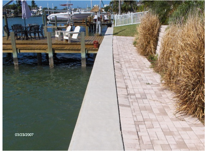
"Bowed" seawall at area below pool.
