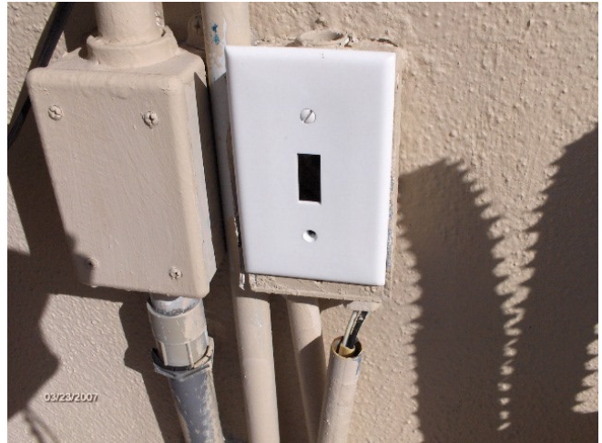
Open junction box with detached conduit to left of patio.
