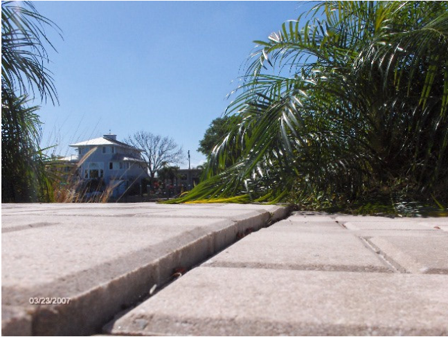
Sunken and separated area of pavers at s/w corner of pool patio.
