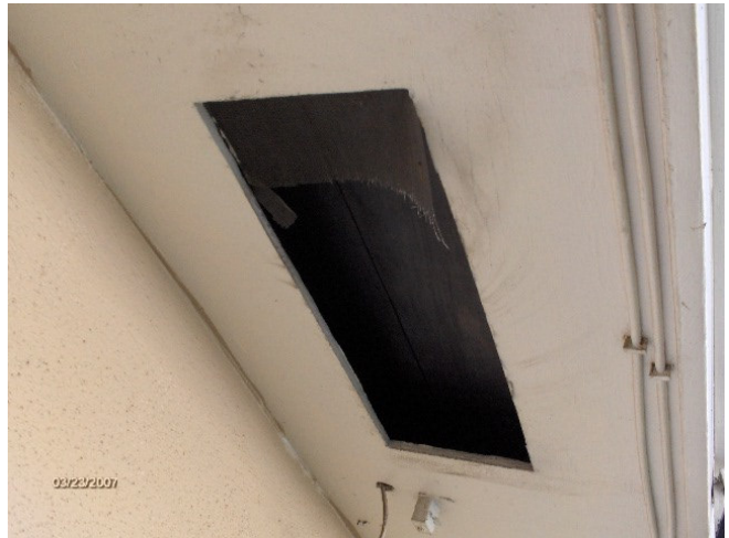
Missing/torn/loose soffit vents at eaves.
