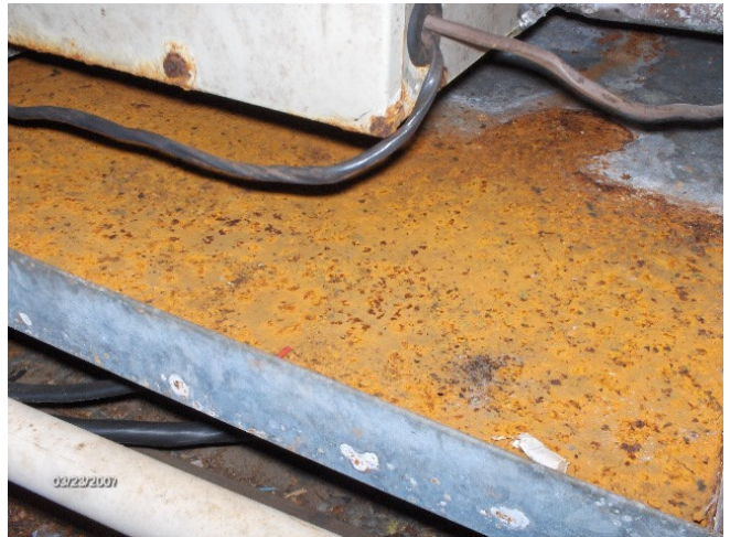
Rust in overflow pan of air handler.
