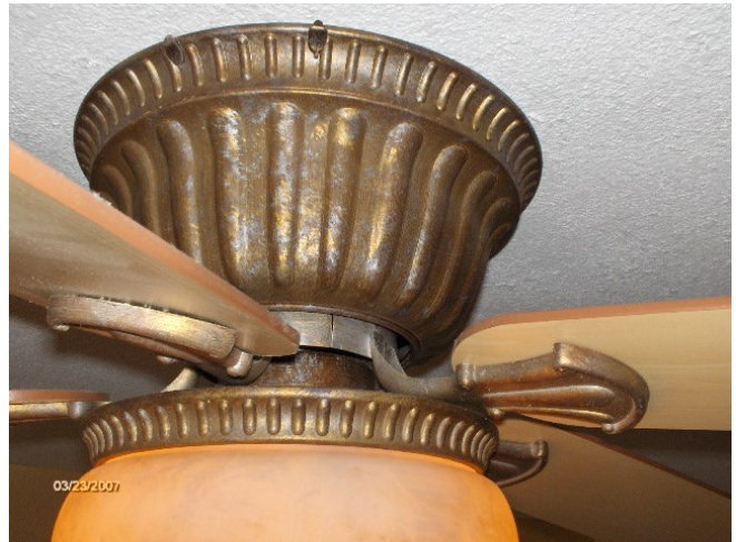
Fan in east bedroom did not operate properly.
