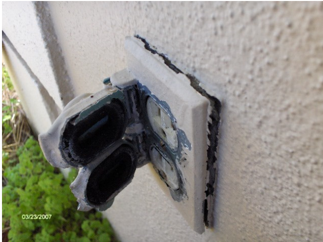
Outlet at n/e corner is loose from wall.
