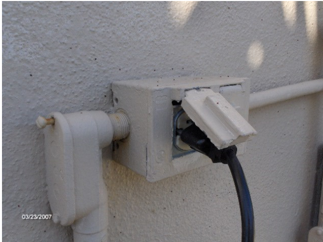
Exterior outlets should have weather resistant covers; most do not.
