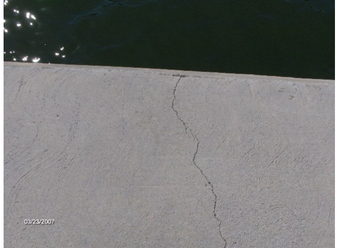
Cracks in seawall.
