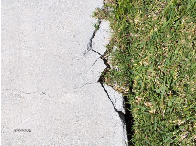
Broken sections of seawall.
