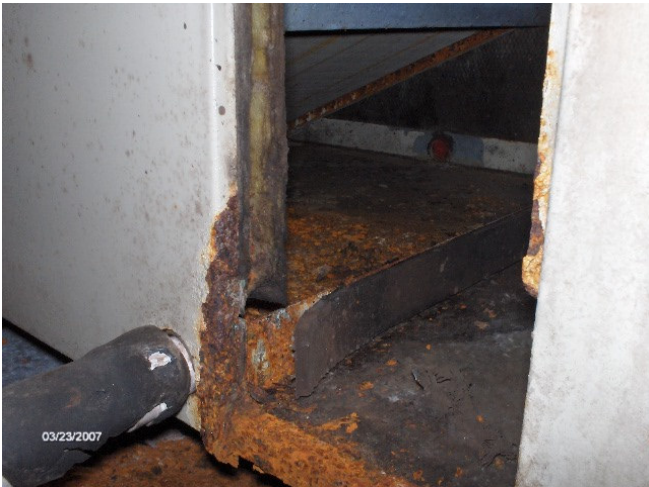
Rust and decay inside air handler.
