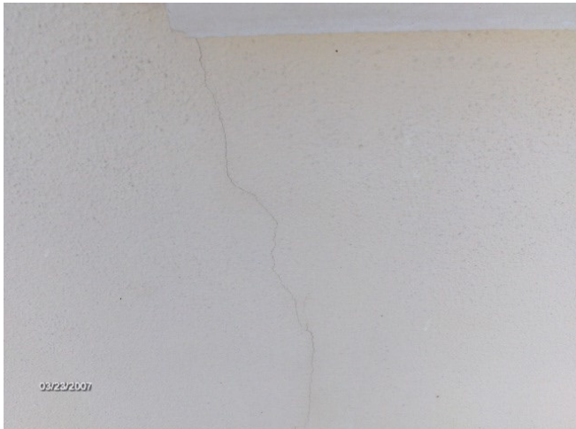
Vertical cracks at s/w corner of stucco wall.
