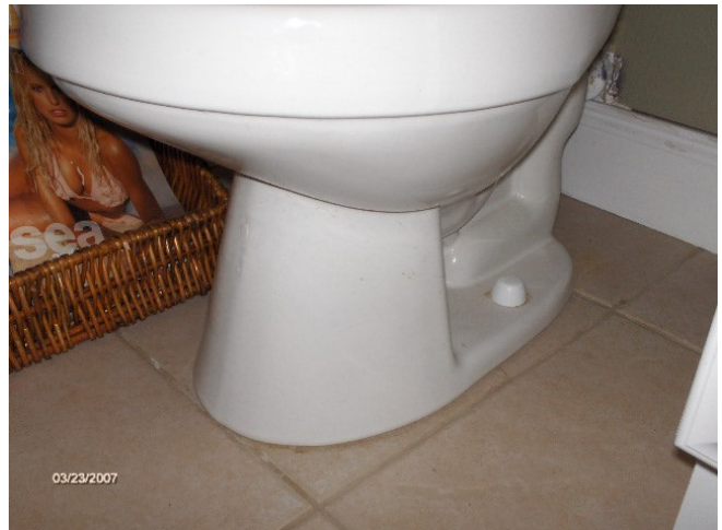
Both toilets in home are very loose from the floors.
