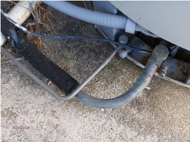
AC freon line missing sections of insulation.
