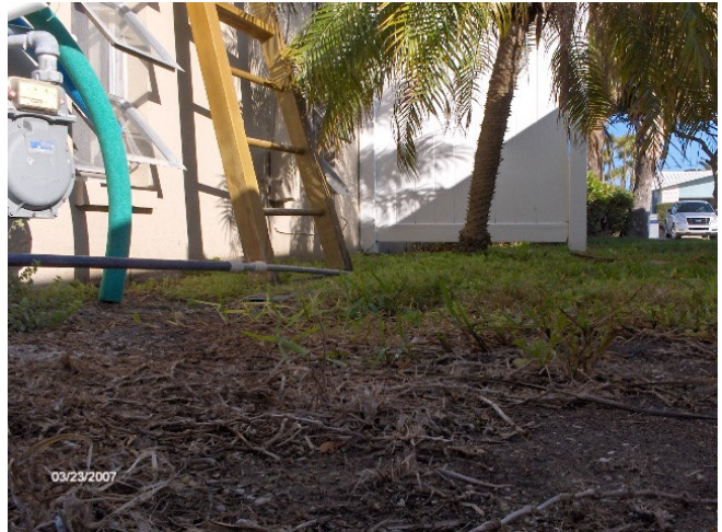
Near level/negative grading at areas of yards.
