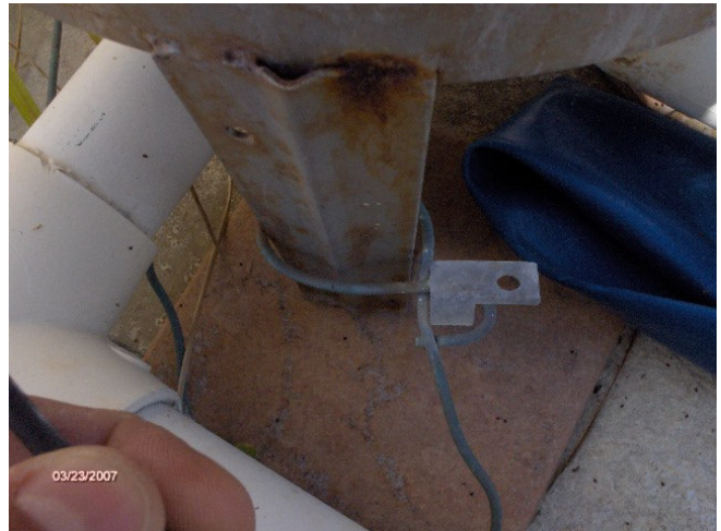
Improper ground at pool filter casing.
