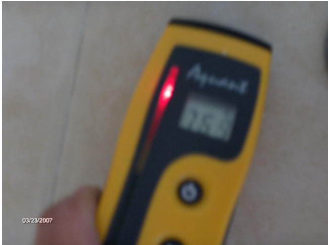
Very high moisture content reading with moisture meter on tilework near faucets of main bathroom shower/tub. See pics below.
