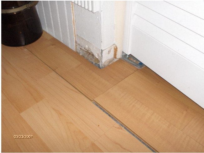
Incomplete molding at several areas of interior.
