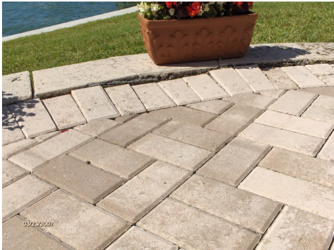
Sunken area of pavers on patio at s/w corner.
