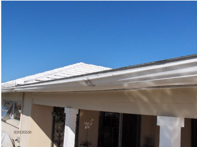
Gutters are misaligned, detached and are missing downspouts and extensions.
