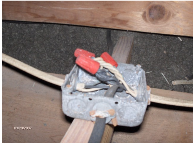
Open junction box in attic access above kitchen pantry.
