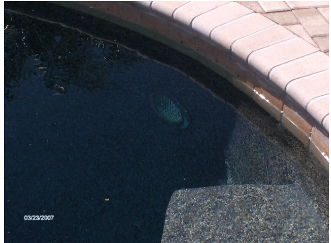
Pool light inoperable.
