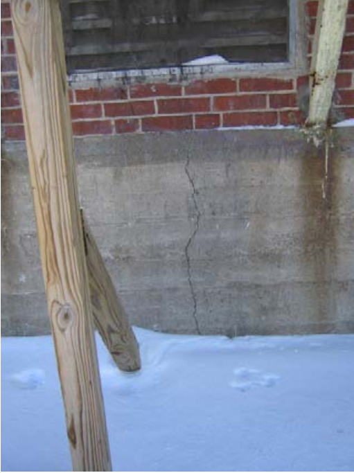
Crack in foundation
