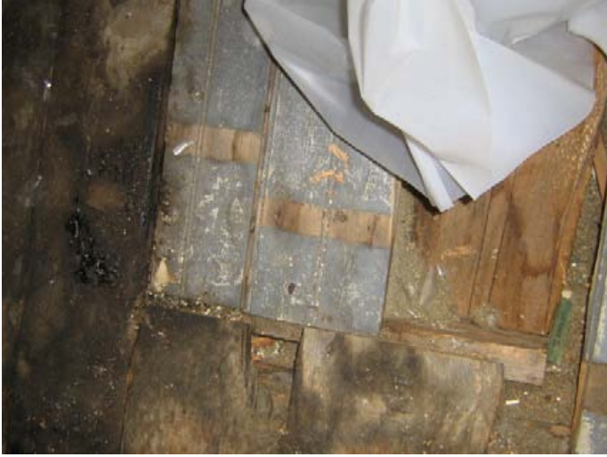
Broken floor boards in attic.
