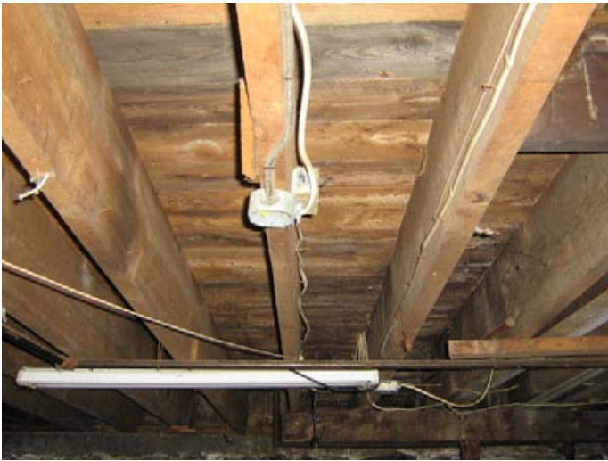
Open junction box
