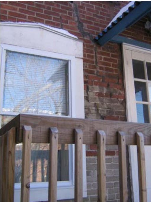
Crack in brick work
