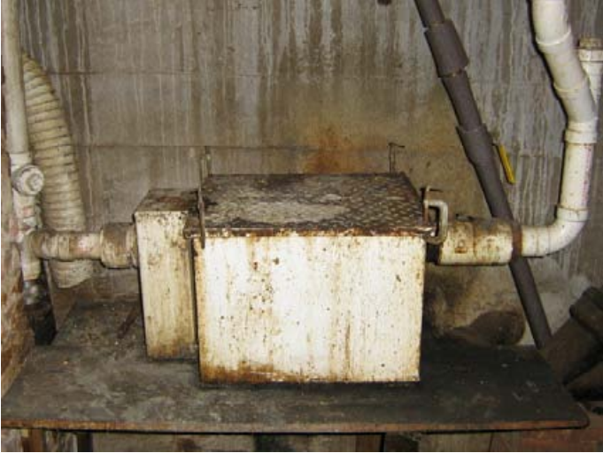
Grease trap in drain line below café.
