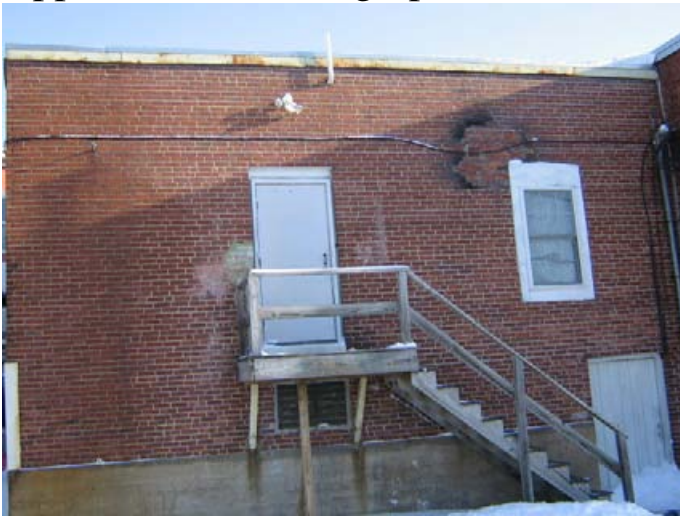
Damage to brick work
