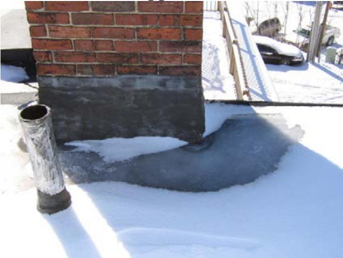
Ice damming around chimney. Area should be monitored.
