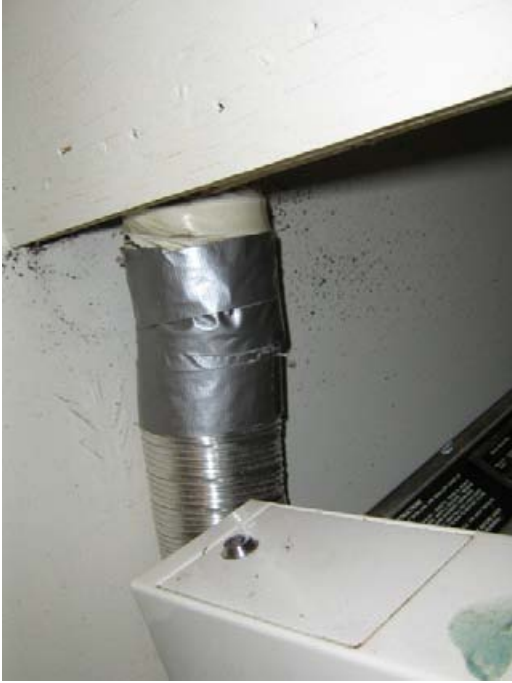
Dryer vent in common hall needs repair.
