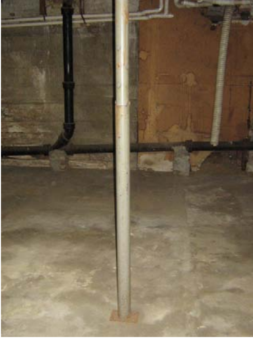
Column in café no footing
