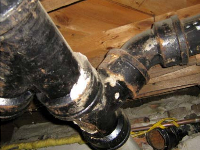
Cast iron septic main line with corrosion.
