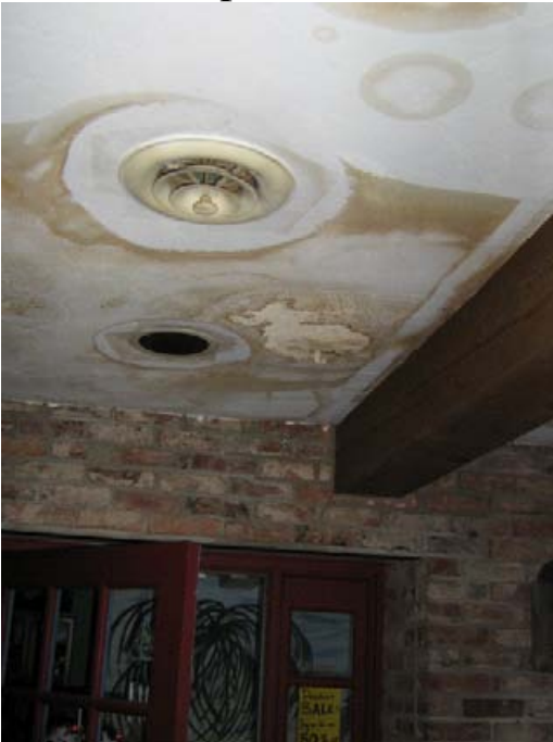
Water stains on ceiling in common hall to tavern and salon.
