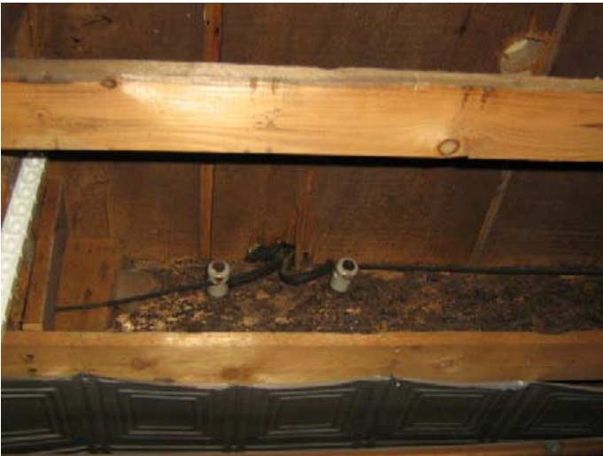
Exposed knob and tube wiring presumed terminated.
