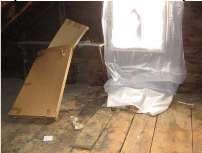
Window in attic with plastic sheeting above apartment # 1.
