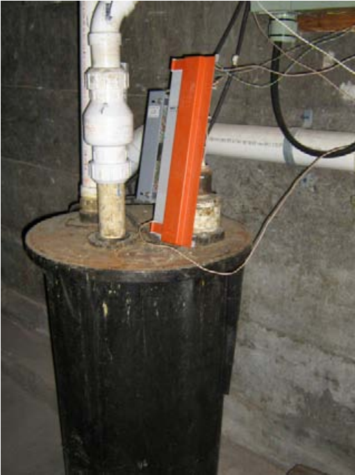
Septic expulsion pump.
