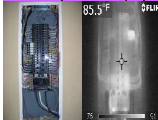
Electrical service panel Infrared image of panel
