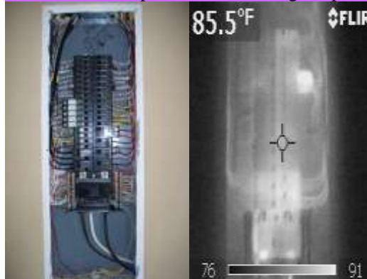
Electrical service panel Infrared image of panel
