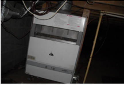
Tankless W/H in crawlspace
