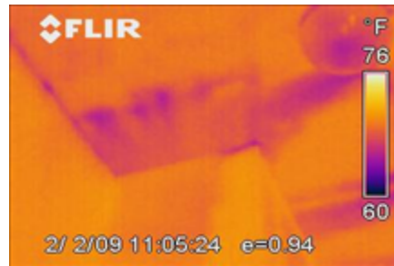
IR image at same ceiling corner
