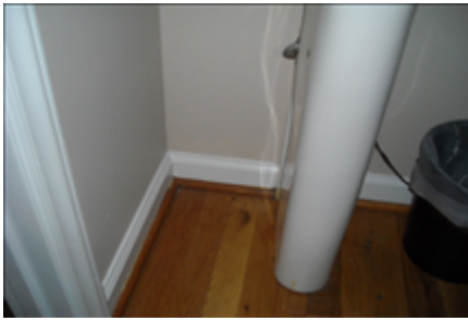
base of interior wall - air flow
