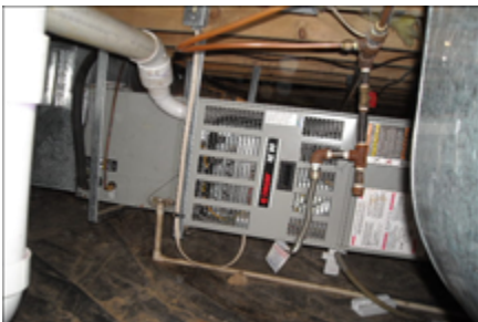
Propane Furnace - Crawlspace
