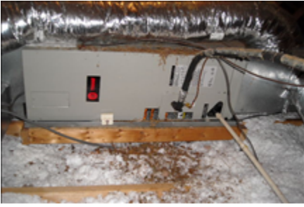
Heat Pump Air Handler - Attic
