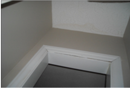
Rt Frt Bdrm closet ceiling
